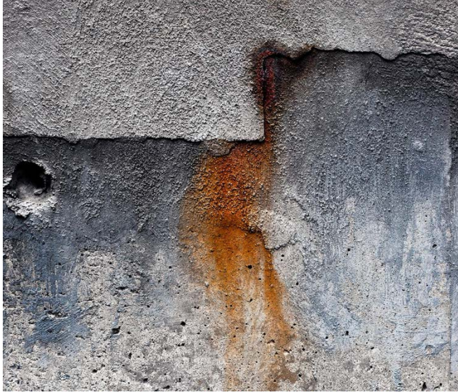
Water damage to a building
